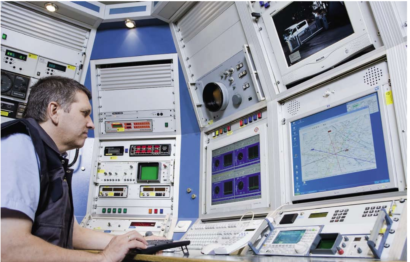
FIG 2 The direction finders and receivers from Rohde&Schwarz in the monitoring stations and test vehicles didn't miss a thing in the complex radio scenario.
